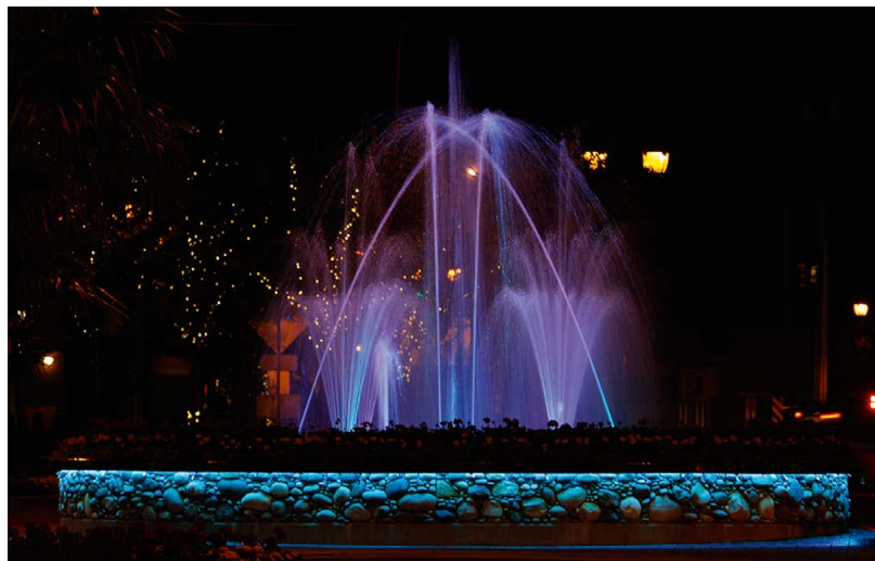
Figure 6: Installation in Langford fountain (Credit: Low Energy Lighting Technologies, EECOL Electric; Photo: The City of Langford)
