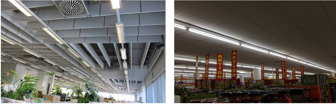
Figure 1: Lamp installations in open office space (left) and supermarkets (right)
