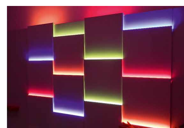
Figure 7: “Wedge Wall” scene settings at the hospitality demo at Osram GmbH, Germany
