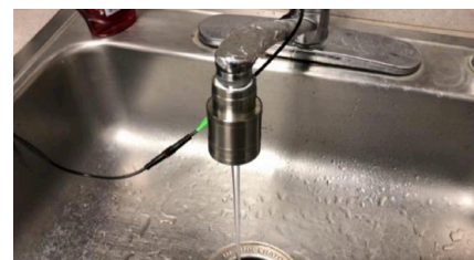
Figure 2: Water faucet (PoU) disinfection.
