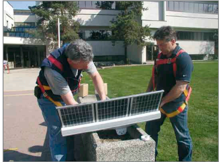
Figure 3: Preparation of the solar engine for installation at the pole by qualified personnel
