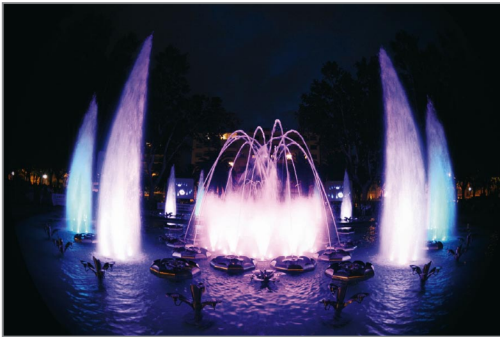
The dramatic illumination of the Perpignan fountain is provided by computer controlled luminaires.
