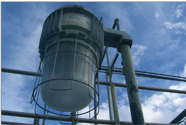
Figure 3: The existing type of lighting fixture used on the installation. This type of fixture is used extensively in the North American market and has been in production for many years.
