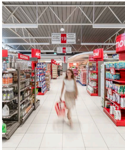
The EUROSPAR grocery store in Lustenau. TECTON luminaires and trunking units were carefully disassembled. These luminaires had been in operation for between four and eleven years at the time this project was launched.
